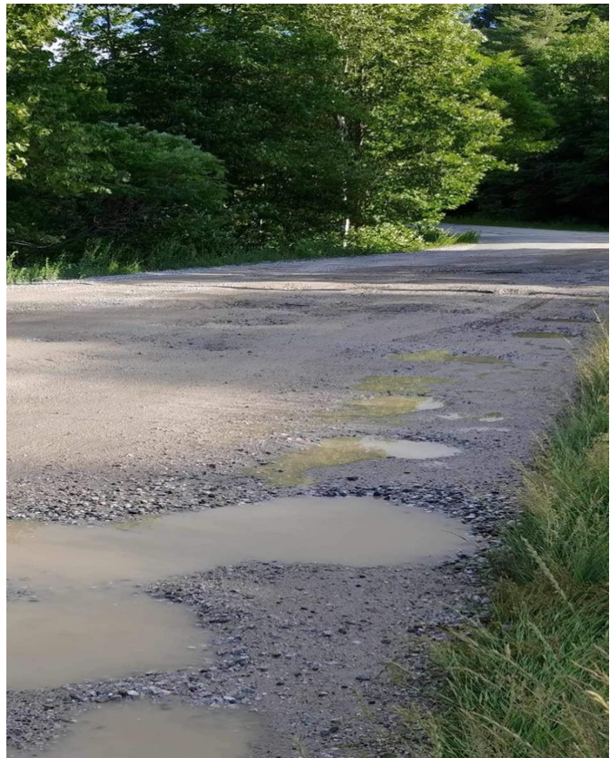
Chemin du Lac Desormeaux in distress. Photos by Julie Bilodeau
